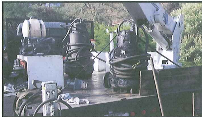
Old Lift Station 1 and 4 Pumps.
