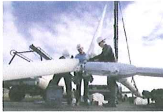
(John Burgess/The Press Democrat) Jesus Ahumada, Greg Tonsil and Rick Van Cleave attach the blades to a wind turbine erected Thursday at the Geyserville sewage pond. The $30,000 turbine will generate power for the sewage facility.
