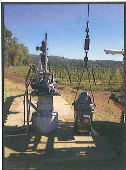
Well 4 pump ready to be installed after receiving routine 10 year maintenance and check-up.
