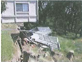
Christopher Chung/ The Press Democrat Damage is shown in April at Jag Singh's home along Lancaster Road in the Lakeside Heights subdivision.
