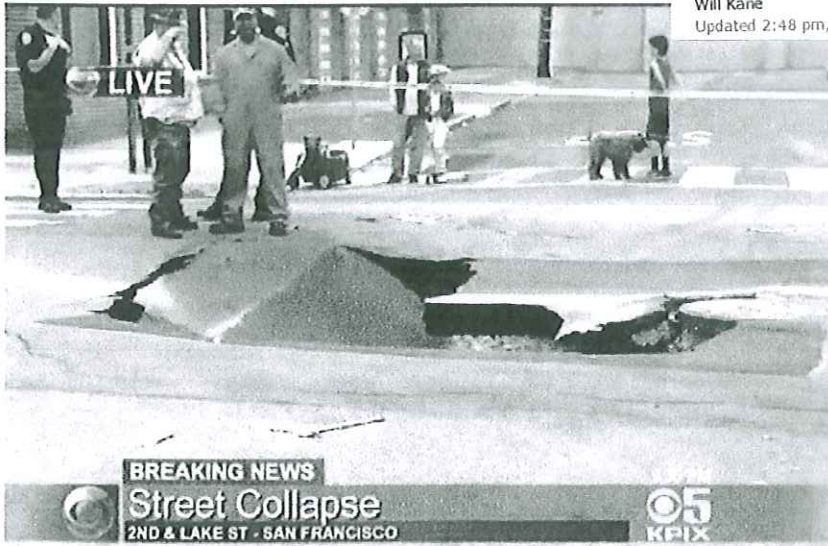
A sinkhole shut down Lake Street and Second Avenue in San Francisco's Richmond District Monday evening. Photo: CBS San Francisco
