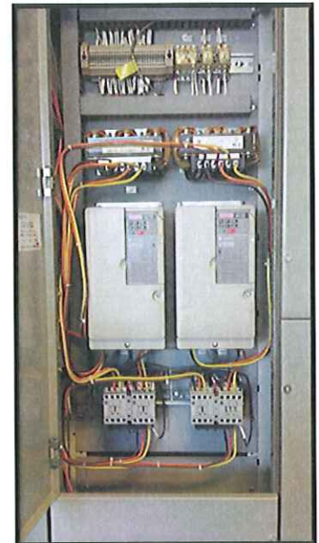
2 variable frequency drives for the Plant Lift Station pumps.
