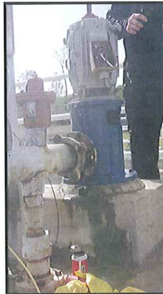
Installation of new Plant Reclaim Water pump. It's used for chlorine motive water, Plant wide hose bibs, and sprays.
