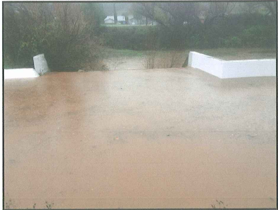
Flood Control during December storm event.
