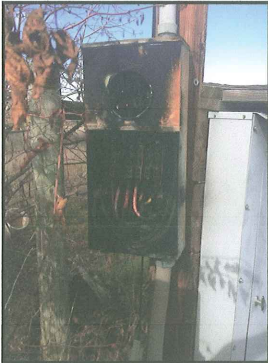
Burnt electrical panel at Well #4.
