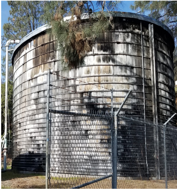
As the Unit 9 tank ages, more leaks occur creating a patchwork of repairs. The darker areas in the above photo indicate continued seepage through the wood.
