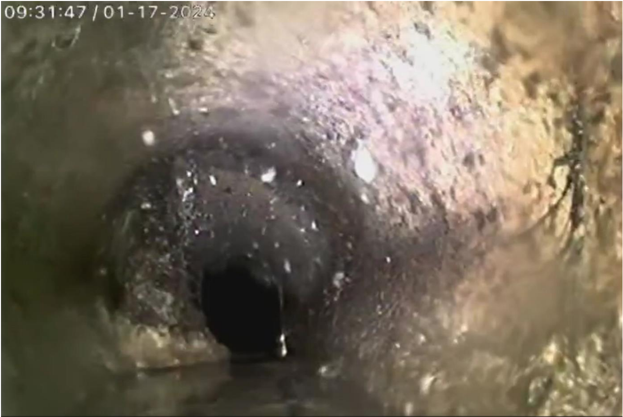
Figure 2. Rootball located at the beginning of the Deer Hill Rd – North Shore Dr easement.
