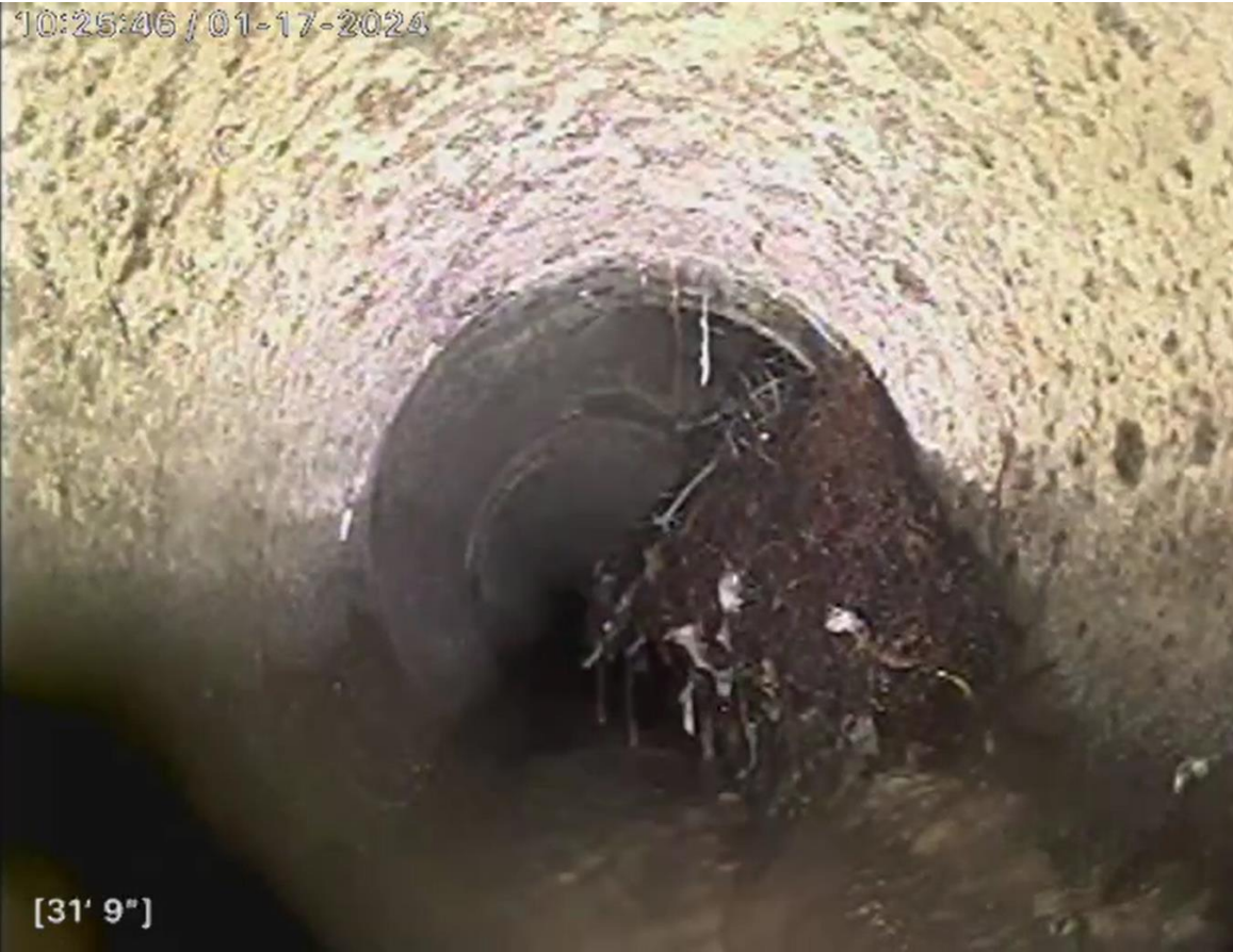
Figure 3. Rootballs from the same lateral found in the sewer main and then on the residential side.
